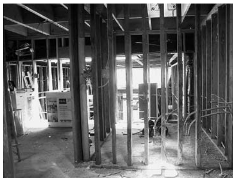
The MEC storefront was remodeled with considerable volunteer effort over a two and one half year period. By the spring of 2005, the renovations were complete and the radio station was on the air full time.
